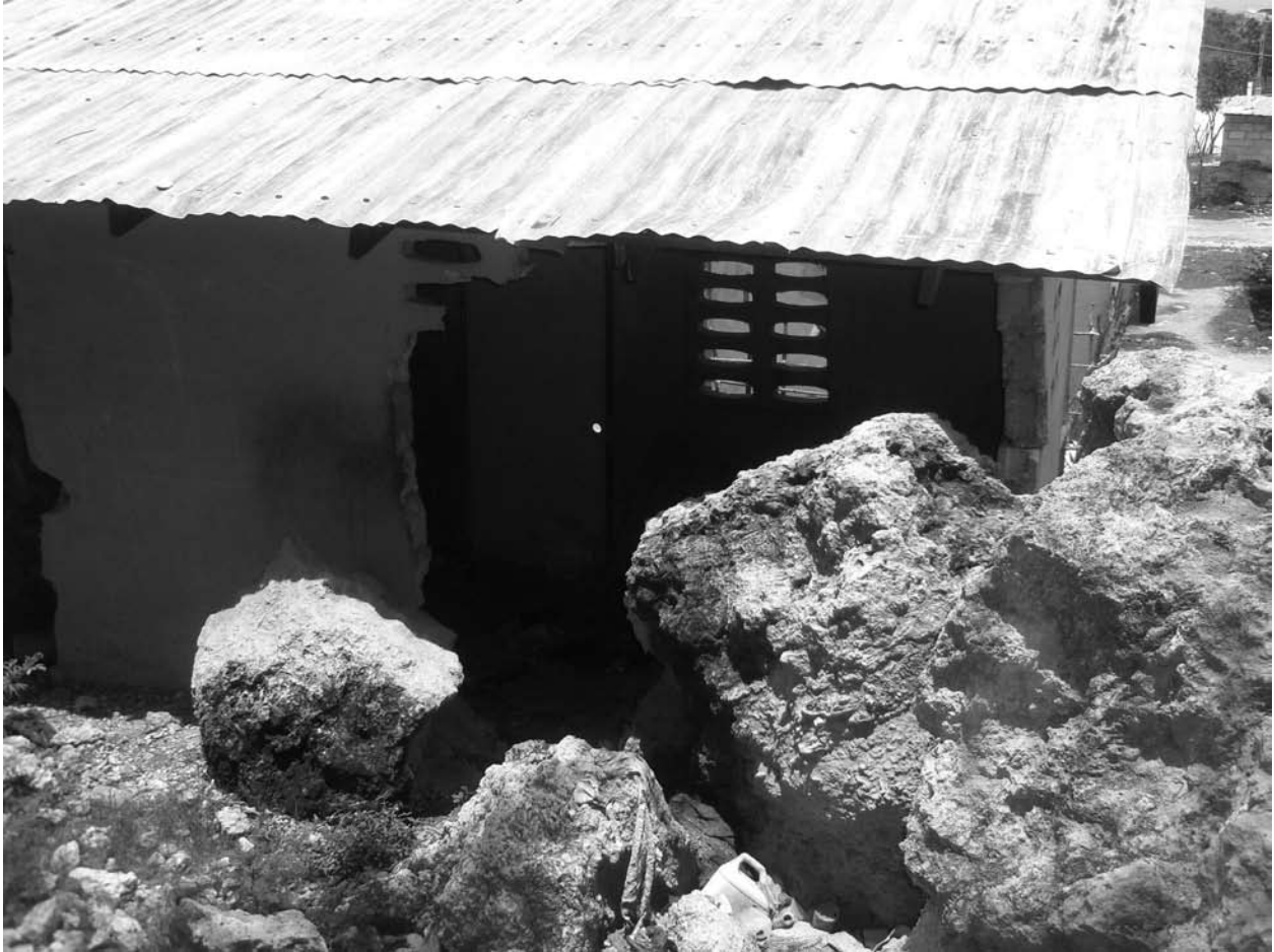
This house, built with assistance from an international NGO, was constructed in an area subject to rock slides.
